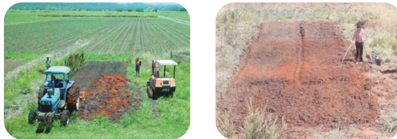
Mixing ViroBind™ reagent into ASS at a sugar cane farm in northern NSW (left) and watering the treating area (right).
