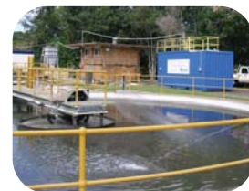
A ViroSewage™ Technology plant in operation.
